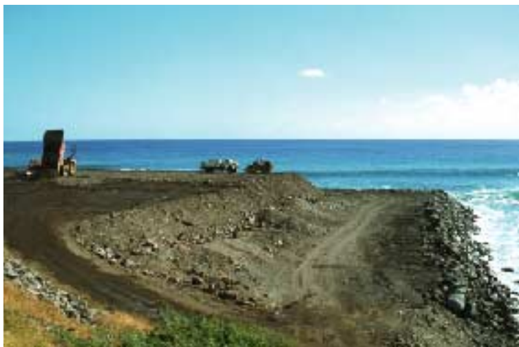
Coastal transformation and artificialization are often major contributors to the deterioration of the subsea environment. (Réunion Island)
