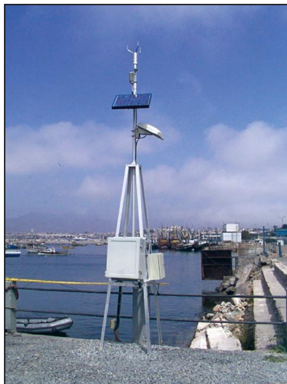
Figure 2. Sea level station configuration.
