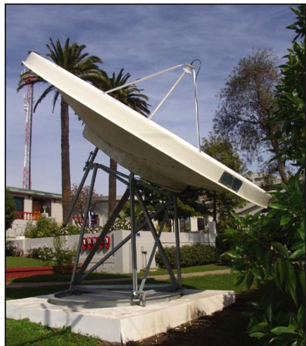
Figure 5. DRGS antenna at SHOA headquarters.
