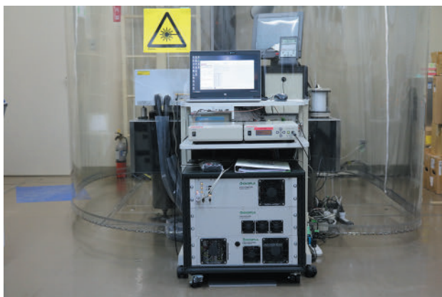
Photo 2. Installed laser oscillator (top) and appearance of the laser system (bottom)
