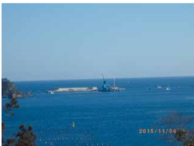
Photo 2. The breakwater at the bay entrance of Ofunato Ko under restoration (taken on November 4, 2015).
