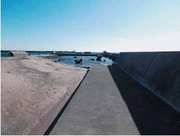
写真 21 b 崩れた護岸 (大津港). Photo 21 b Destroyed seawall (Otsu Harbor).
