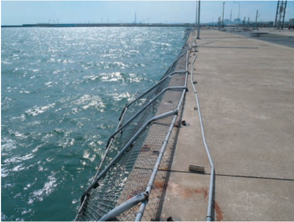
写真 11 a 倒れたフェンス。 Photo 11 a Fence which fell down.
