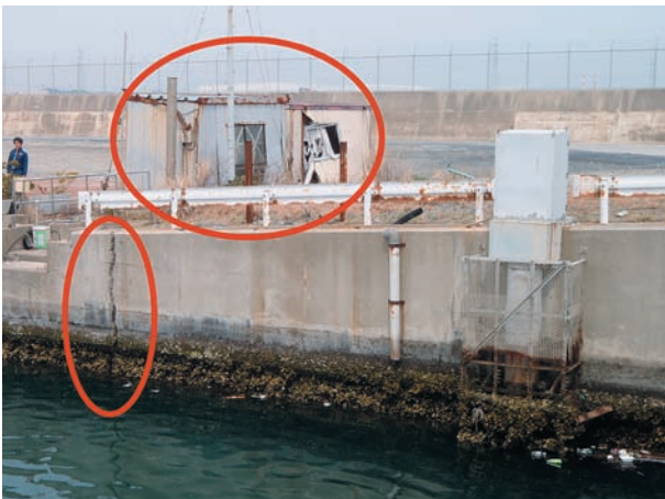
写真 13 a 岸壁の亀裂と崩れたプレハブ. Photo 13 a Rift in a quay and a destroyed prefab.
