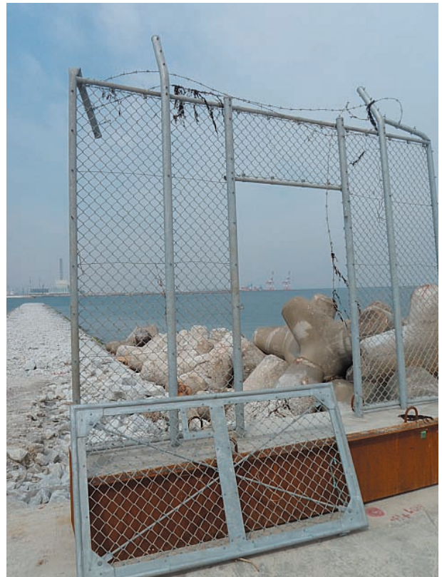
写真 13 c 倒れたフェンス. Photo 13 c Fence which fell down.
