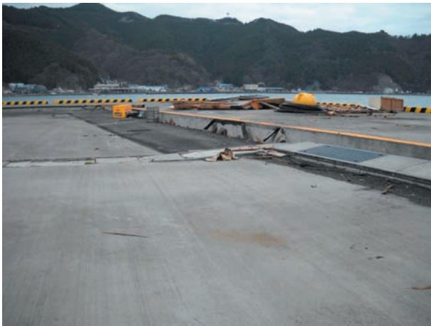
写真 3 a 沈下したふ頭. Photo 3 a Wharf which subsided.
