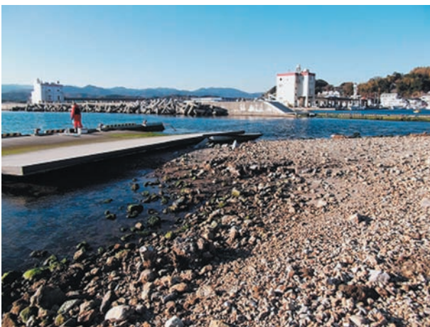
写真 21 d 崩れた護岸 (大津港). Photo 21 d Destroyed seawall (Otsu Harbor).
