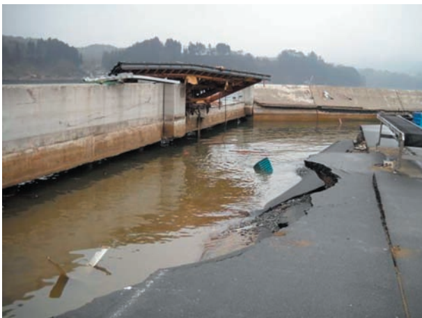
写真7c 気仙沼港石油栈橋。 Photo 7 c Oil pier in Kesen-numa Harbor.
