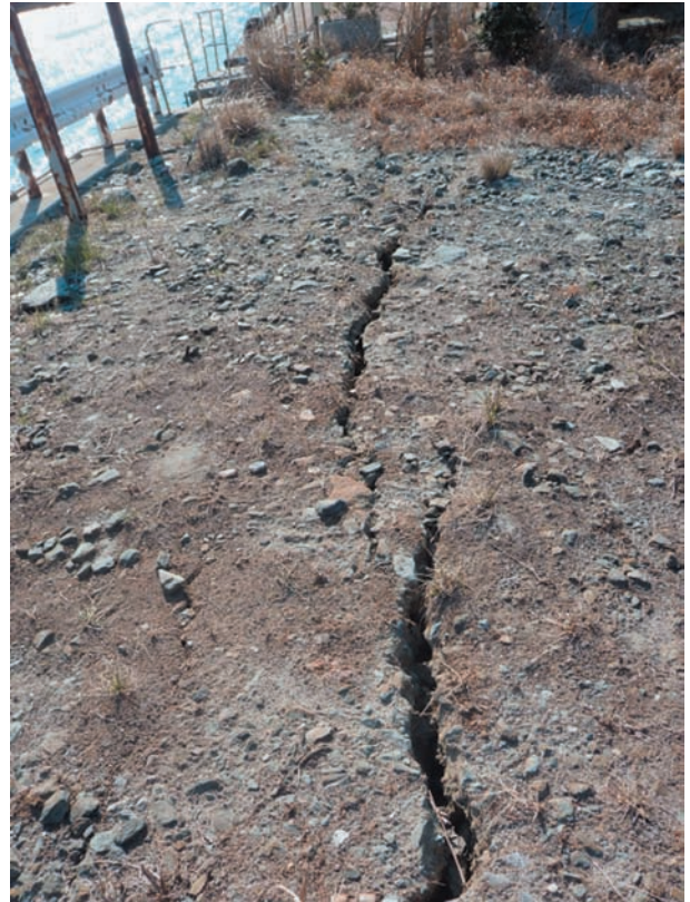
写真 13 b ふ頭の亀裂. Photo 13 b Rift in a wharf.
